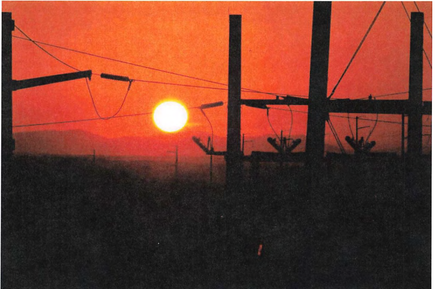
Electrical infrastructure at sunset.
